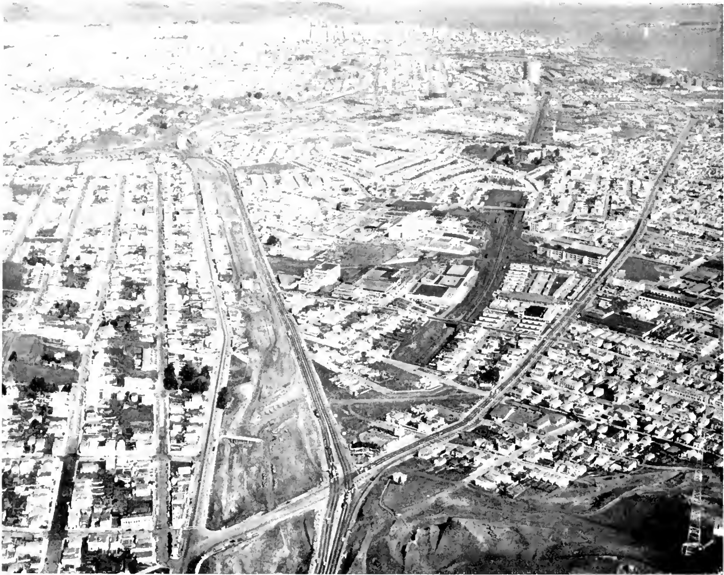
View of construction progress on Bayshore Freeway in San Francisco from Third Street looking toward Alemany Boulevard
